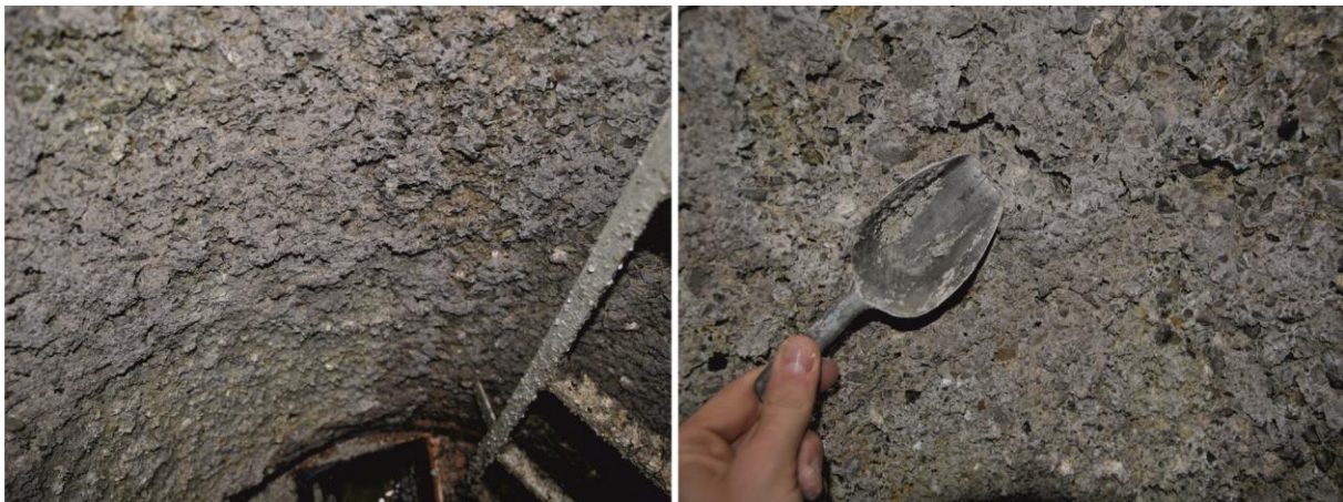
Figure 4: Strong deteriorated concrete in one of the manholes of the first gravity sewer section.
