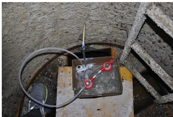
Figure 16: Gas trap in a corroded manhole. This trap consists of two “Woulf’sche bottles” that contain 5% Zn-acetate solutions and an air pump. Here, H 2 S reacts with the Zn-acetate to form solid ZnS.
