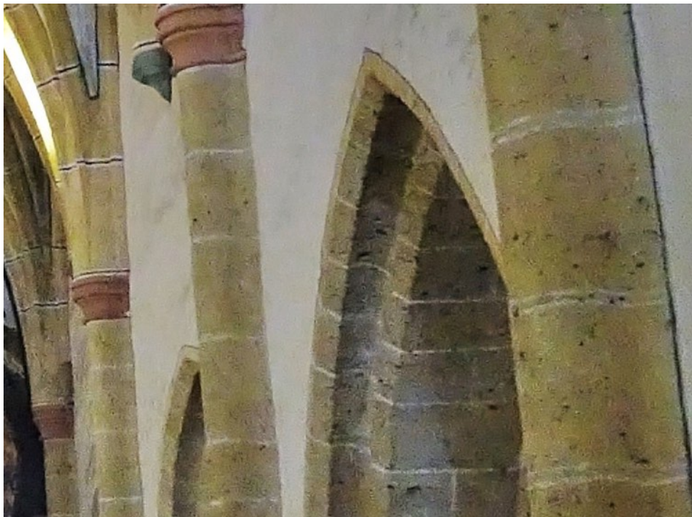
Figure 47: Archway with holes due to fallen out pebbles.
